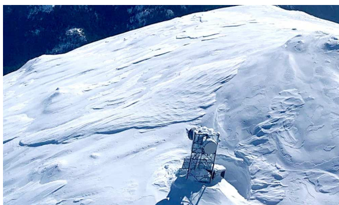
Sunfire-Remote 400 powered microwave radio station in Alaska
