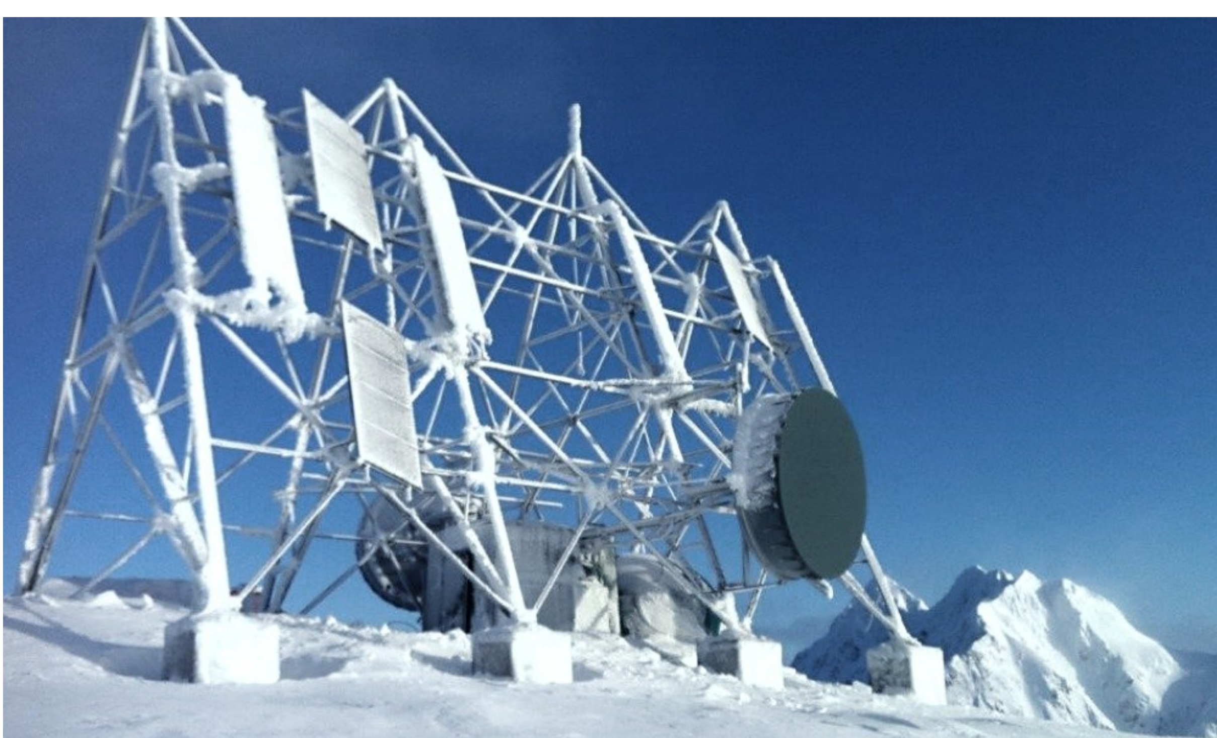
Sunfire-Remote 400 powered microwave radio station in Alaska
